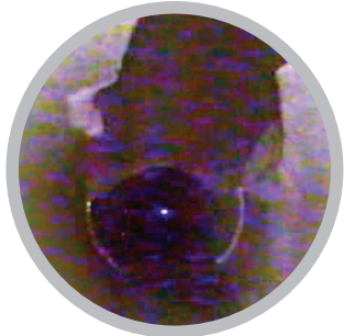
Broken / Missing Pipe
